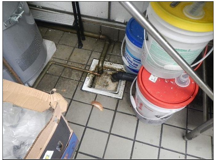
14. Floor sink or drain in tenant kitchens
