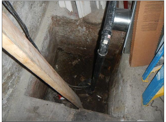
8. Sump in basement
