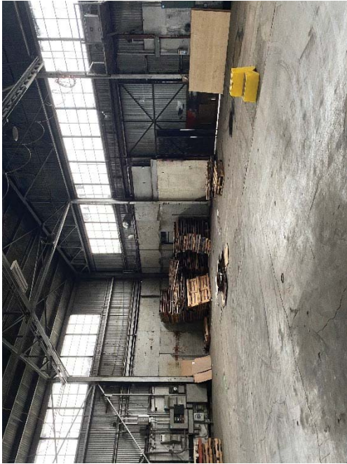
Photo 3: Stained floor in the northeast corner of the 703 Bancroft Way building.
