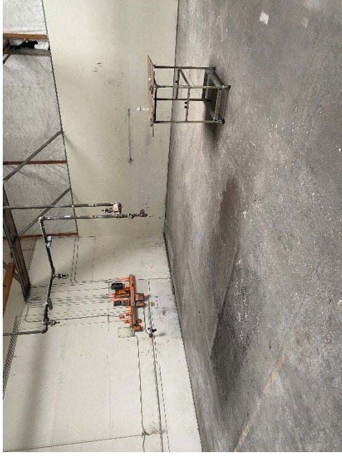
Photo 14: Staining on the floor of the former Ironies Fabrication building.
