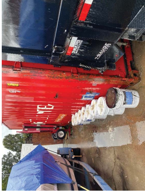
Photo 8: Paint and sealant containers stored in the parking lot adjacent to the 705 Bancroft Way building.
