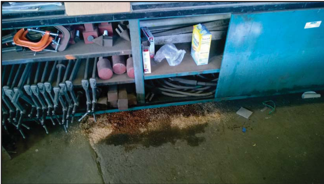
Oil staining around base of work bench.
