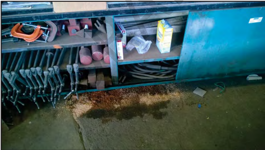
Oil staining around base of work bench.
