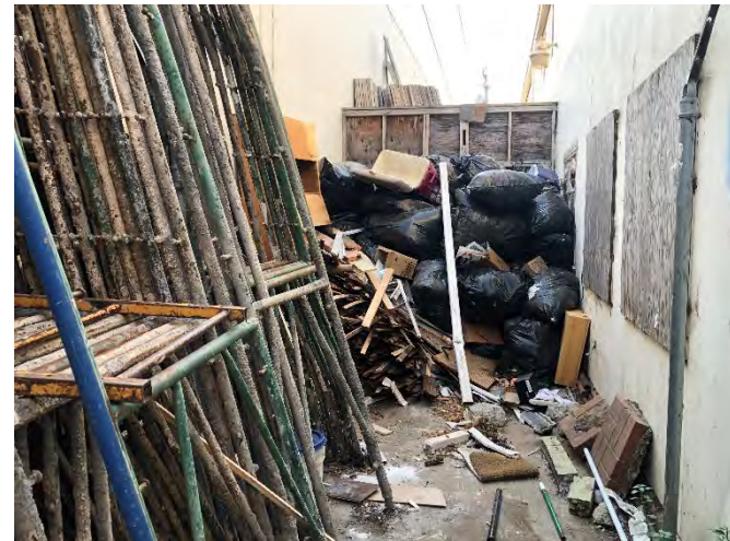
Photo 28: Trash and debris located on the west side of the 705 Bancroft Way building.
