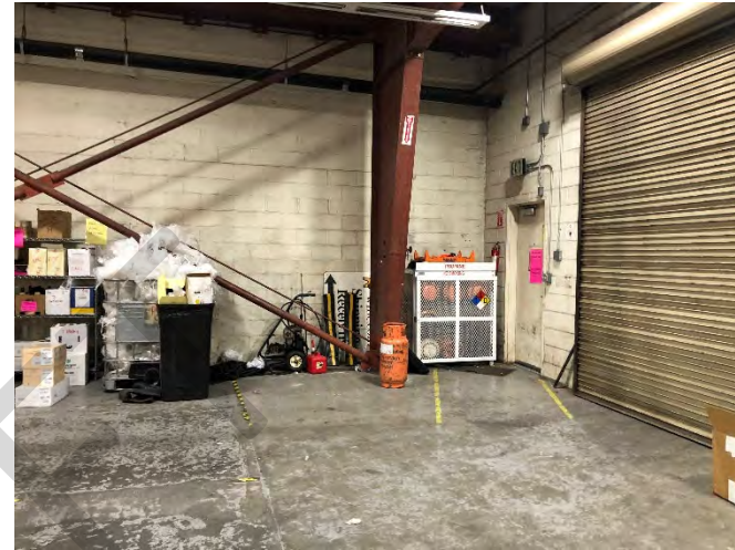
Photo 2: Propane storage area located at the north end of the WINE.COM warehouses (2200 Fourth Street).
