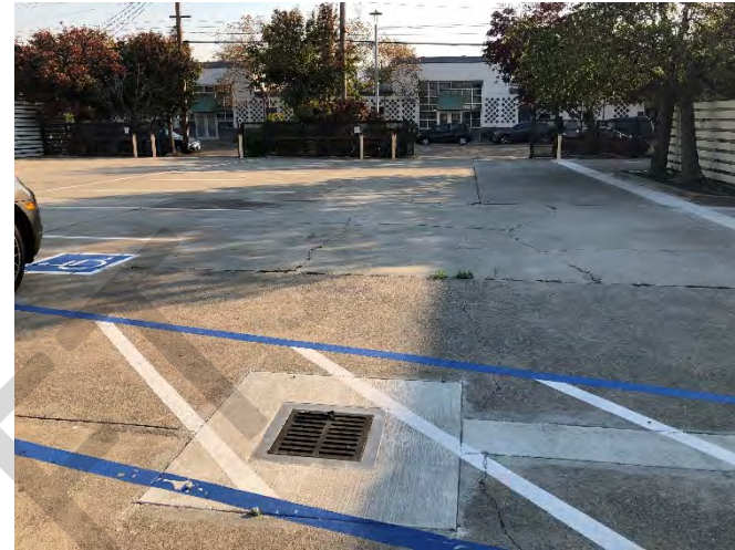
Photo 18: Storm drain located in the parking lot of the former Acuity Brands Lighting facility.
