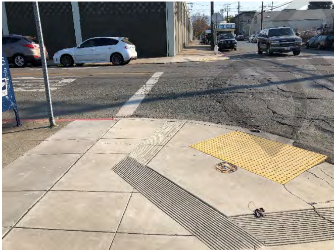
Photo 35: Groundwater monitoring well located on the corner of Bancroft Way and Fourth Street.
