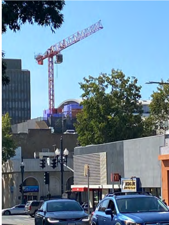
LEFT High rise construction crane in downtown RIGHT New high rise on University Avenue and Shattuck Blvd
