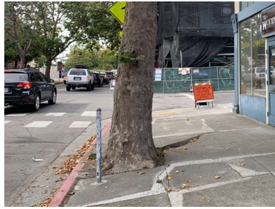
Figure 27. Many existing sidewalks are in poor condition.
