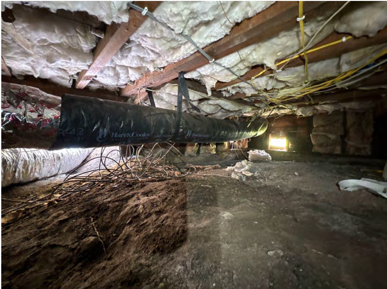
Caption: The crawlspace of a home receiving a ducted mini-split.
