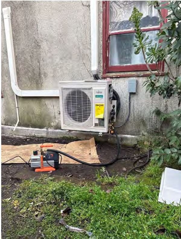
Caption: A heat pump installation with its connected lineset and service disconnect.
